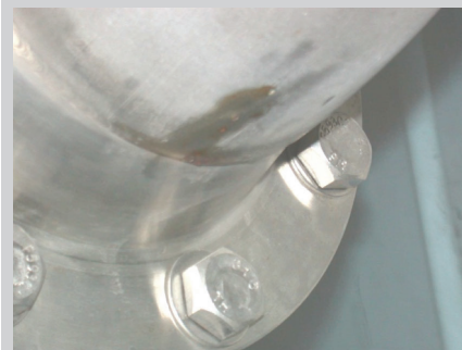
Fig. 2. Acidic fumes in the glovebox exhaust contributed to the corrosion in this extract ductwork.
